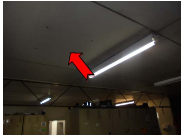
Photo 4. Interior, ground level, change room, ceiling – asbestos-containing fibre cement sheeting.
