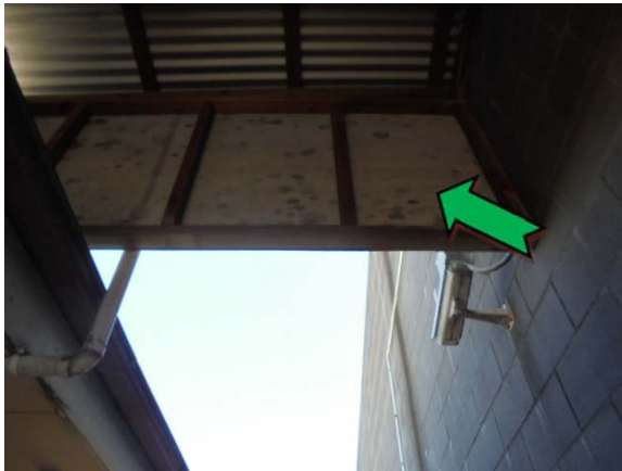
Photo 3. Exterior, western elevation, Infill panels high level – non asbestos-containing fibre cement sheeting.
