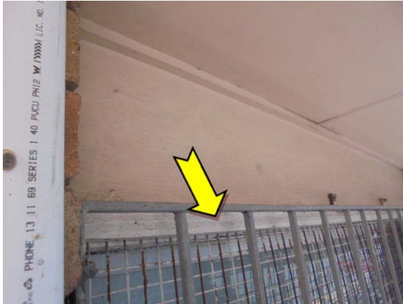
Photo Exterior, throughout, window frames – 7. suspected lead-containing white upper paint system.
