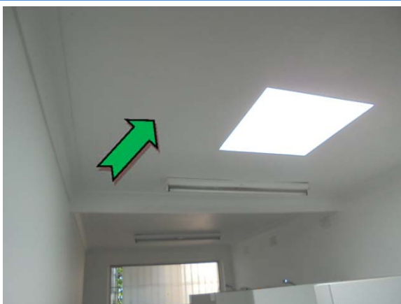
Photo 5. Interior, ground level, Shower and male toilets, ceiling – non asbestos-containing fibre cement sheeting.
